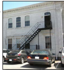
Fire escape in violation of current building code
