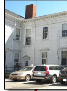
Hanging disconnected wires
