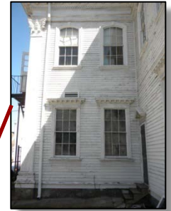
Decrepit hardscape, plant growth through foundation
