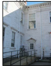
Ramp not up to current ADA and MAAB standards
