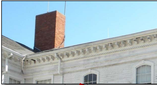
Broken and missing dentils
